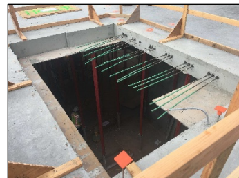
Stairwell opening where workers had recently removed a plywood cover.
