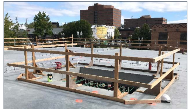
Stairwell opening the framer fell through.
