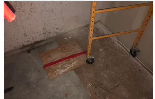
Photo 2: Unsecured plywood cover over the open floor hole.
