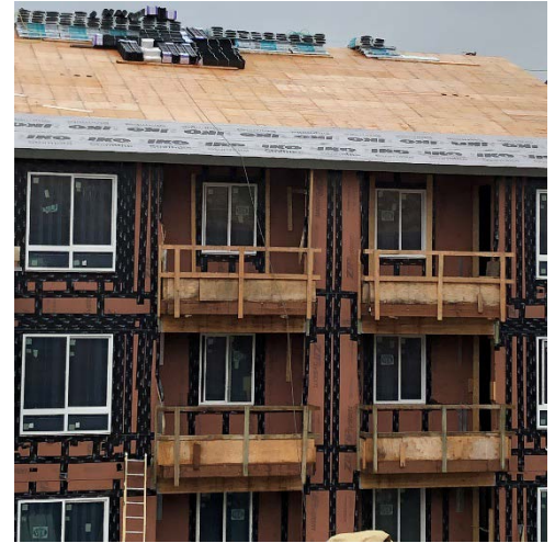
Three-story apartment building from which the roofer fell 30 feet.
