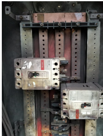
Service panel breakers after the arc flash explosion.
