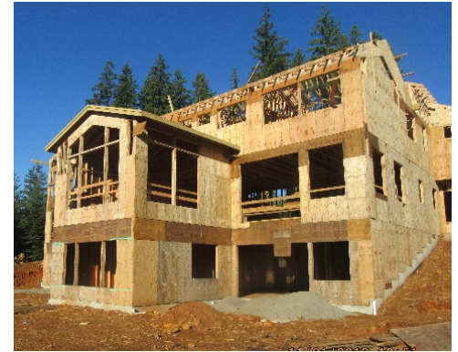
House where framer fell 25 feet from the lower back sheathed roof. He was not using fall protection.
