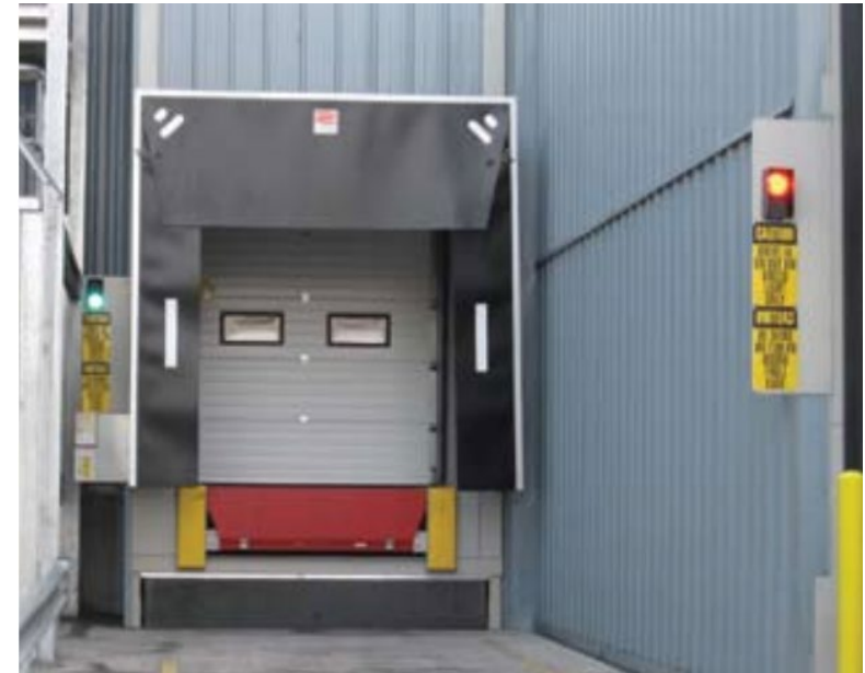
Photo 6: Loading dock with bay door seal, warning signs, and traffic signal-style vehicle movement indicator lights. Photo courtesy of Freight Transport Association.
