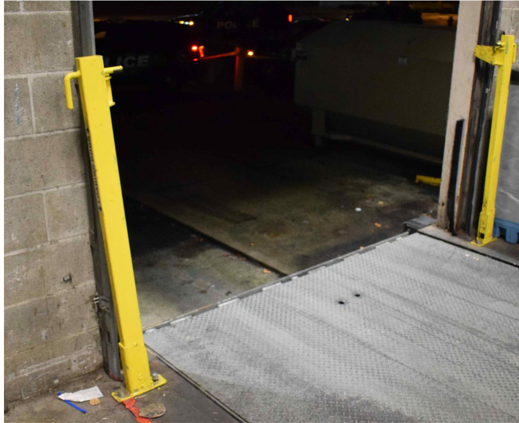
Photo 3. Interior view of loading dock where incident occurred. The injured clerk fell to the driveway outside after being crushed by the trailer against the exterior wall.
