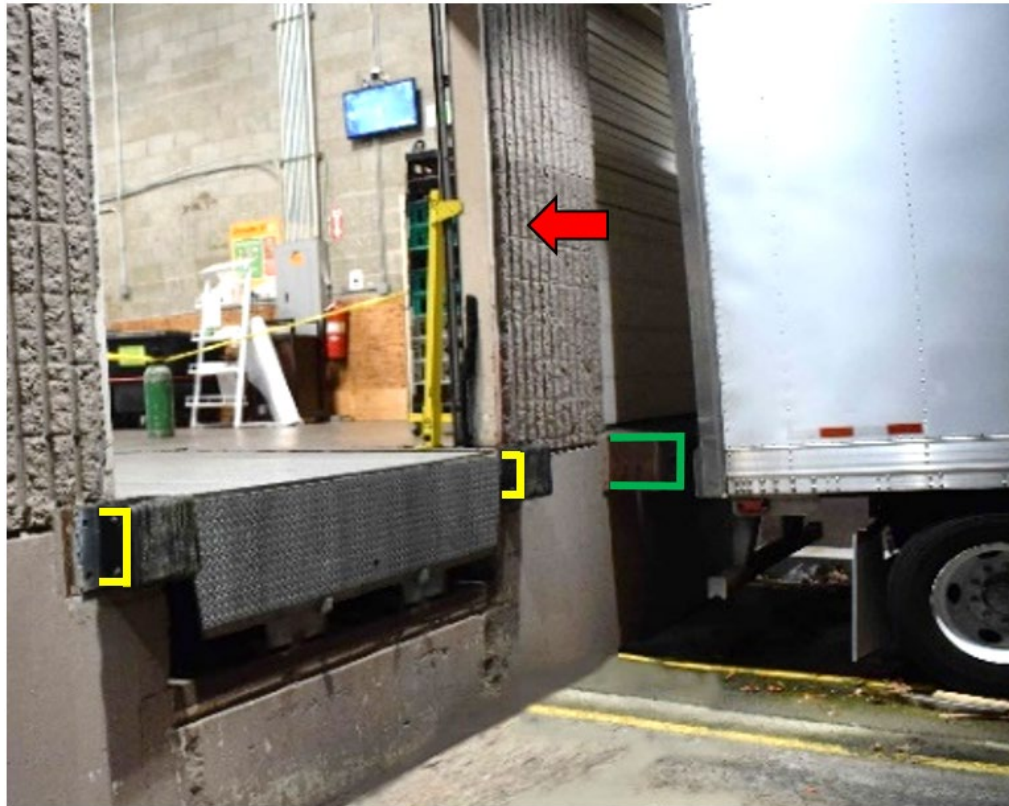
Photo 2. Red arrow shows where clerk was crushed while leaning through a gap between the exterior wall and rear of the trailer. The gap resulted from the trailer being parked several inches away from the yellow-outlined 6-inch deep dock bumpers, possibly to make space to unfold the dock leveler lip. The green outlined dock bumpers at the loading bay on the right were larger.
