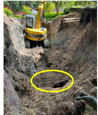
The yellow circle shows the ditch inside the trench where the contractor and laborer were buried.
