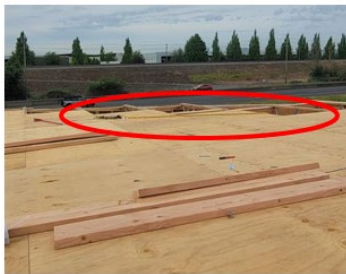
Fall protection anchor, shock-absorbing lanyard, and lifeline near leading edge where worker fell.
