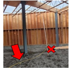
Lifeline with rope grab stretched to show excess length from worker's fall location (x).
