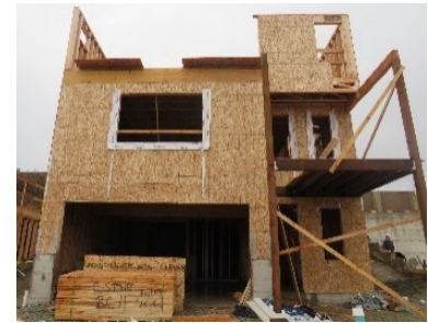
Open-sided upper floor where guardrails were removed.
