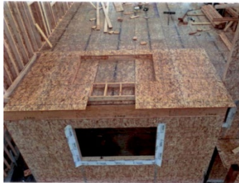
Unprotected floor where the framer fell.
