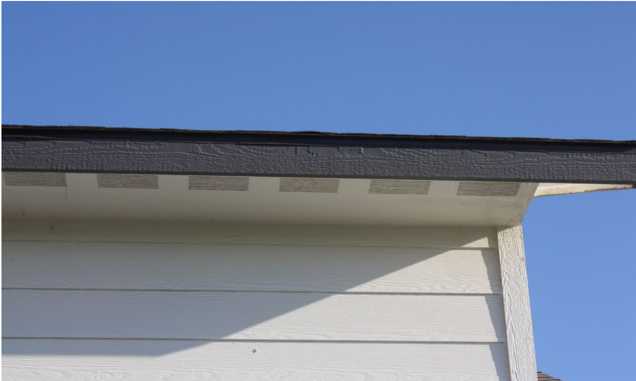
Photo 2. Upper roof above the patio where the installer was prying when he fell.
