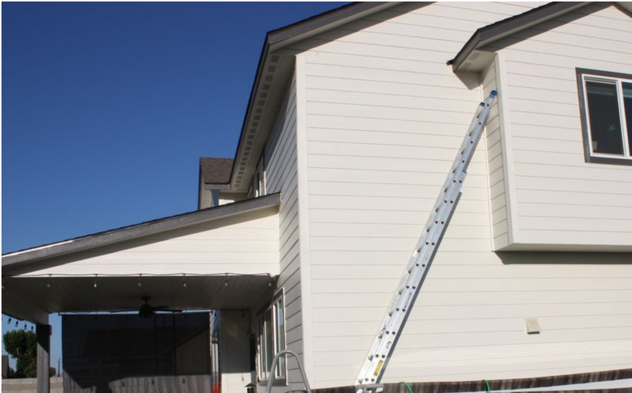
Photo 3. Edge of the patio roof where the installer was working and from where the fell, opposite from where the ladder was propped.
