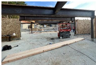
Fallen wooden beam and second lift at incident site.
