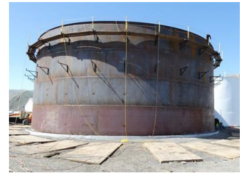
Storage tank at incident site.
