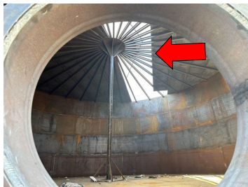
Hole in roof where welder fell.
