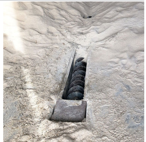
Sub-floor auger that the worker was entangled in with guards removed after rescue effort.
