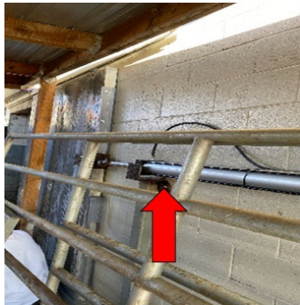
Wall-mounted pneumatic cylinder that actuated door.
