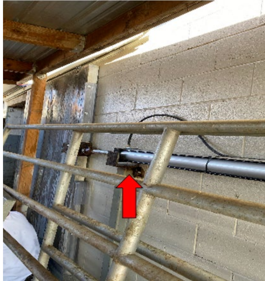
Photo 5. Wall-mounted pneumatic cylinder that actuated door.
