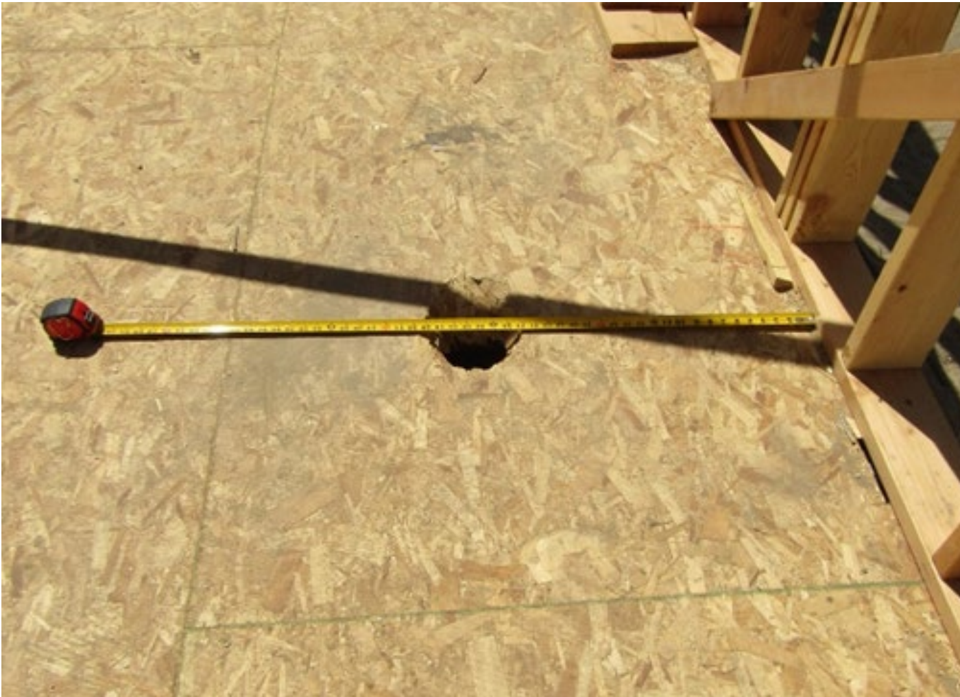
Photo 2. Hole in \frac{3}{4} -inch decking is from the impact of the framer's head.
