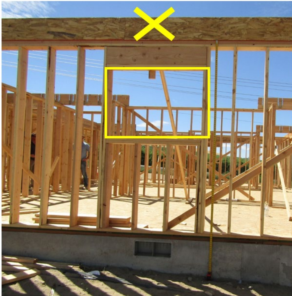
Photo 1. Framers fell from rim joist (x) above window opening to floor deck.
