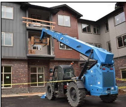
Scene where worker fell.
