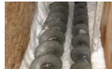
Photo 2: Danger Area: Don't enter spaces with exposed double-screw conveyers until you verify the equipment has been properly locked and tagged out.
